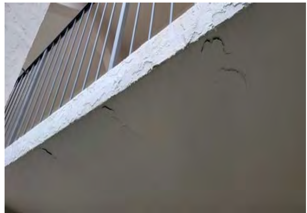
54 Cracked Walk Near Unit 106
