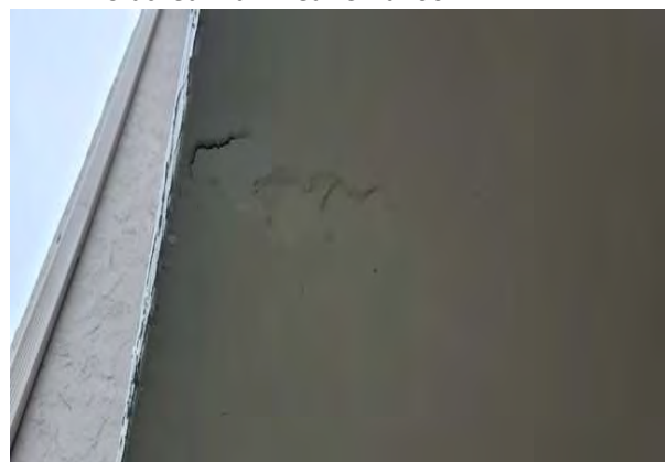
56 Cracked Walk Near Unit 106
