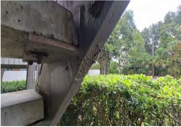
88 Rusted Stringer 2nd Floor to 1st Floor at Left Stairs
