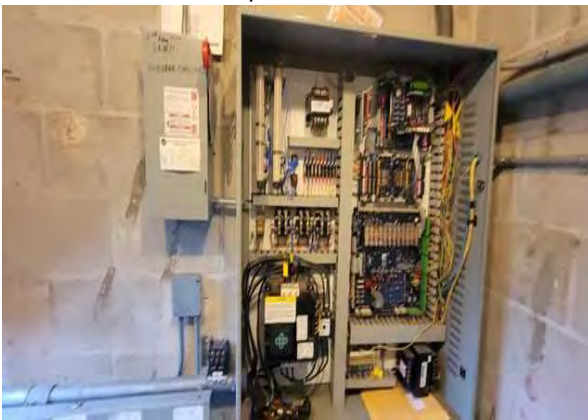
13 Elevator Control Board
