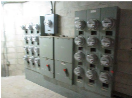
15 Electrical Meters & Main Panels
