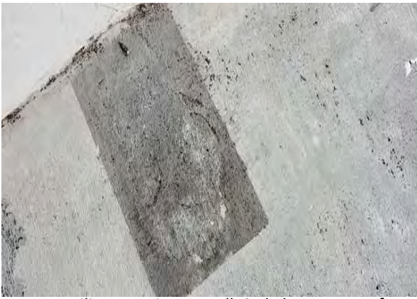
89 Failing Repairs to Walk 3rd Floor Near Left Stairs
