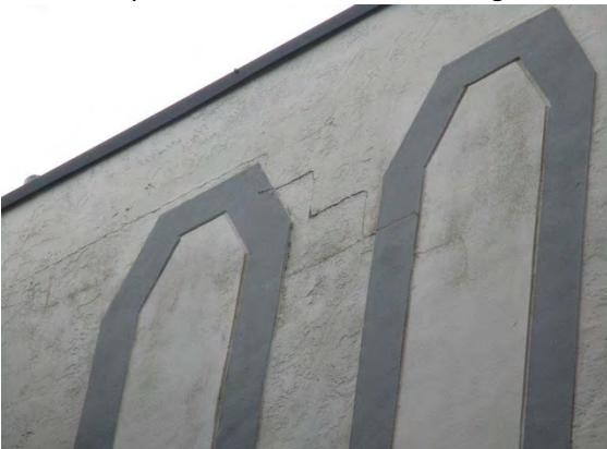
31 Moderate Step Crack With Displacement Rear of Building
