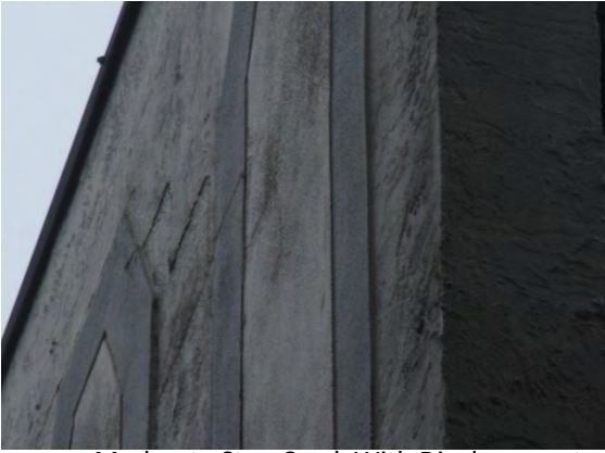
33 Moderate Step Crack With Displacement Rear of Building
