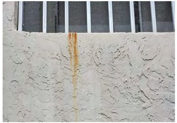
42 Unit 202 Rust at Balcony
