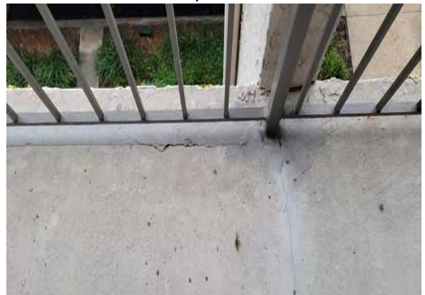
45 Crack in Walkway Near Unit 304
