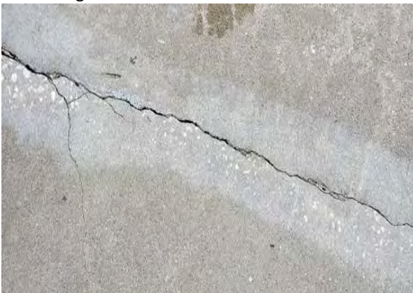
54 Crack in Walkway Base of Stairs 2nd Floor Right Side
