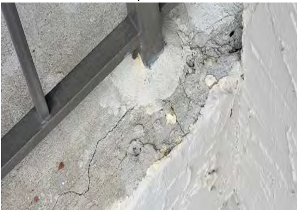
36 Cracked Walkway Near 303
