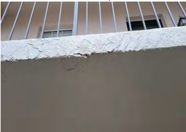
45 Cracked Walk Above Unit 102
