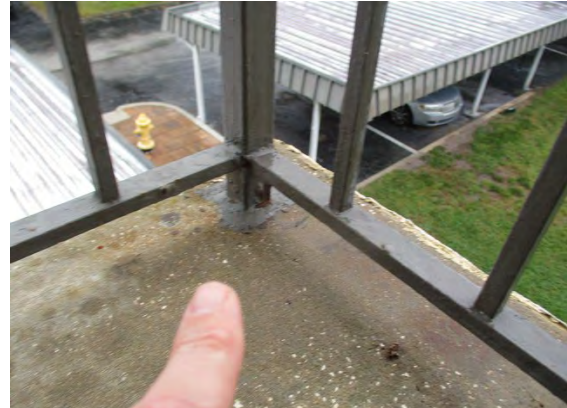
6 3rd Floor Railing Corroded In Multiple Areas
