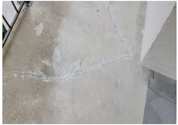
74 Cracked Walk Multiple Areas 2nd Floor
