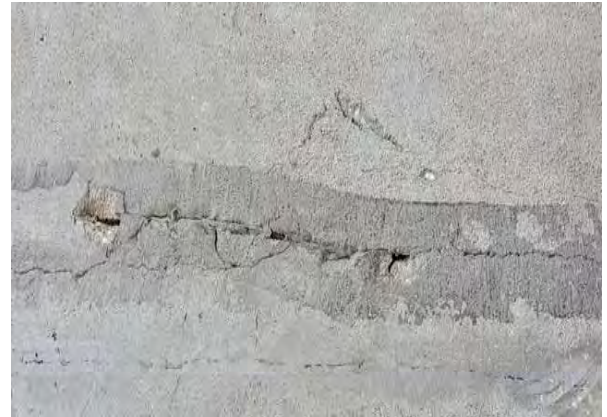
35 Cracked Walkway Near 303 Exposed Rebar
