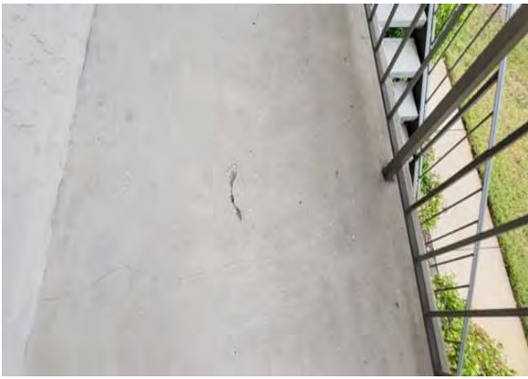
56 Spalled Concrete 2nd Floor Near Right Stairs
