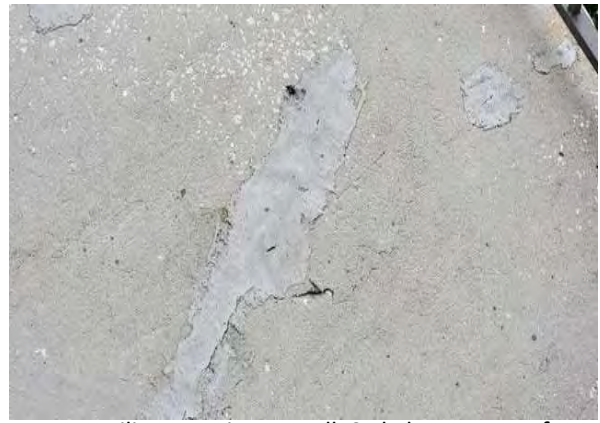
90 Failing Repairs to Walk 3rd Floor Near Left Stairs
