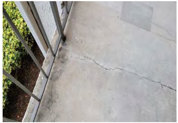
65 Crack in Walkway Near Unit 205
