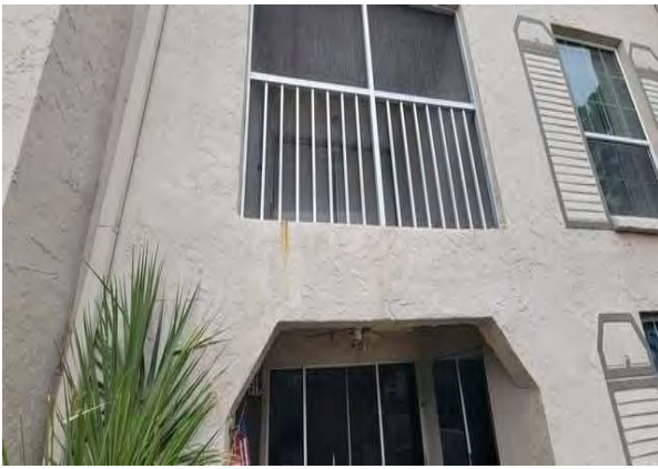
41 Unit 202 Rust at Balcony
