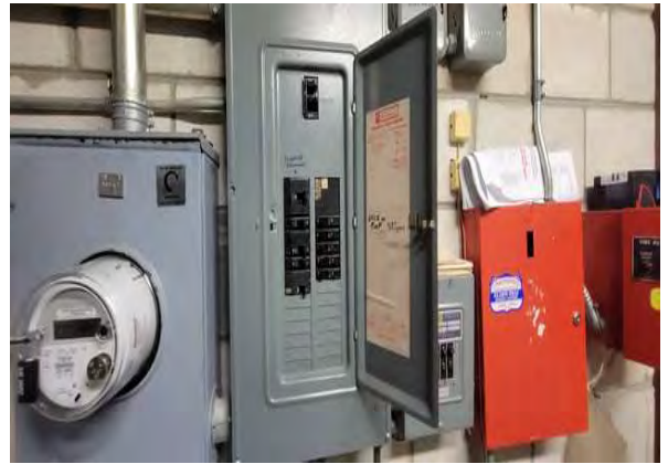
14 Electrical Room Panel
