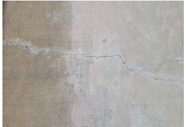
76 Cracked Walk Multiple Areas 2nd Floor
