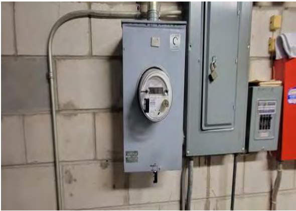
13 Electrical Room Meter
