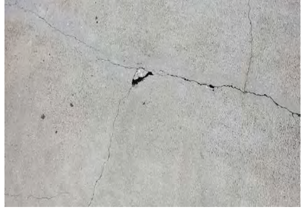
71 Crack in Walkway Near Unit 204
