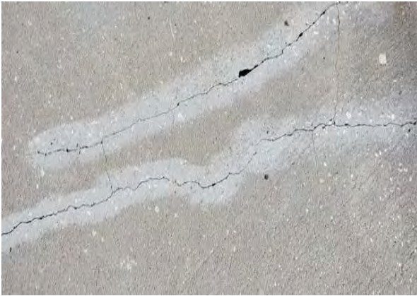
50 Crack in Walkway Near Unit 306
