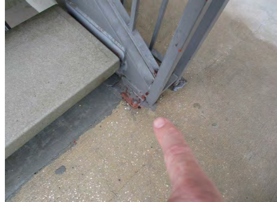
28 Right & Left Stairwells Corroded At Connection Points
