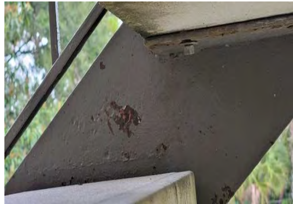
85 Rusted Stringer 2nd Floor to 3rd Floor at Left Stairs
