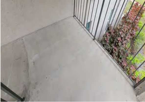
67 2nd Floor Right Staircase Cracked Walk
