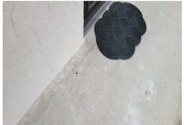
104 Spalled Concrete Near Unit 305
