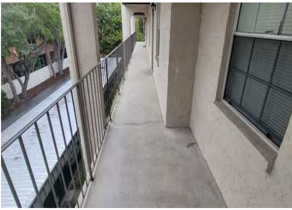
32 Cracked Walkway Near 303
