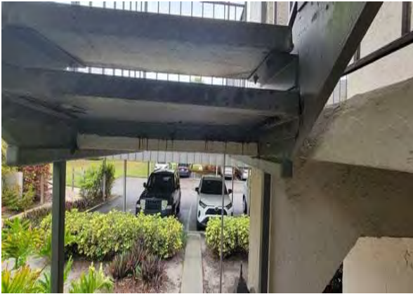
59 Rusted Right Staircase 1st Floor
