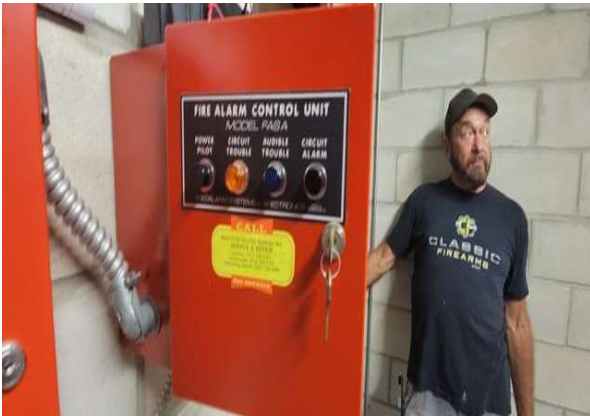
15 Fire Alarm Control Unit
