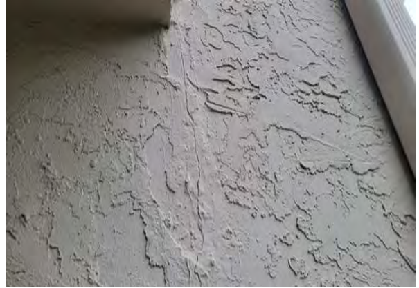
52 Crack in Wall Near Unit 103
