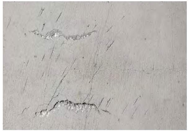
66 2nd Floor Right Staircase Spalled Concrete
