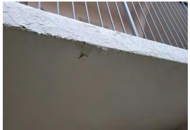
48 Cracked Walk Above Unit 102
