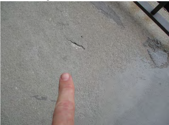
15 3rd Floor Walkway Concrete Spalling Multiple Areas
