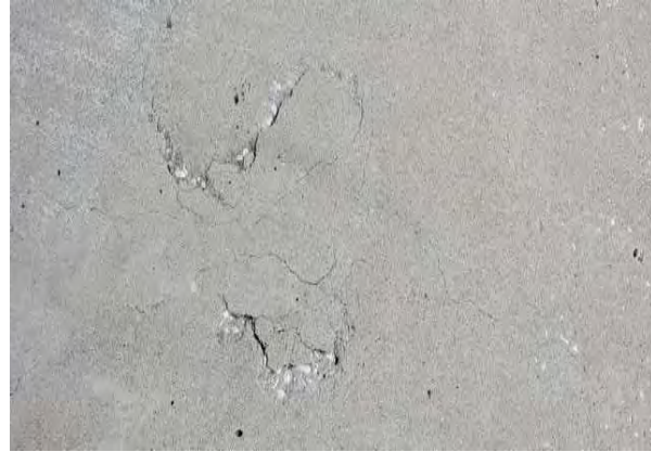
92 Spalled Concrete Near Unit 301
