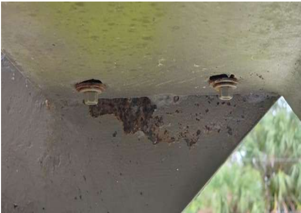
84 Rusted Stringer 2nd Floor to 3rd Floor at Left Stairs
