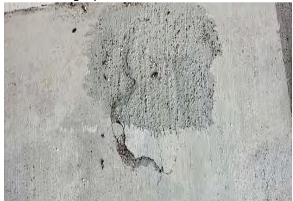
88 Failing Repairs to Walk 3rd Floor Near Left Stairs
