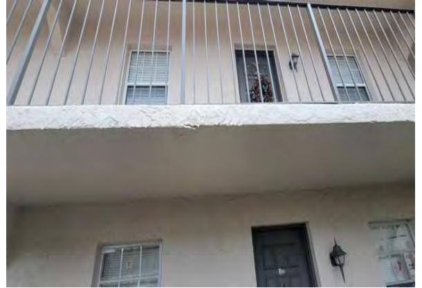
44 Cracked Walk Above Unit 102
