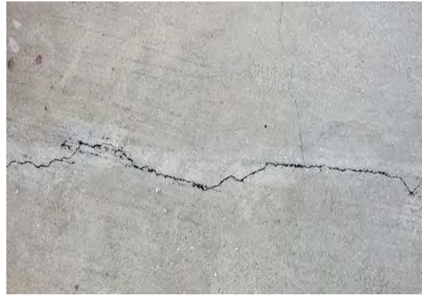
67 Crack in Walkway Near Unit 205
