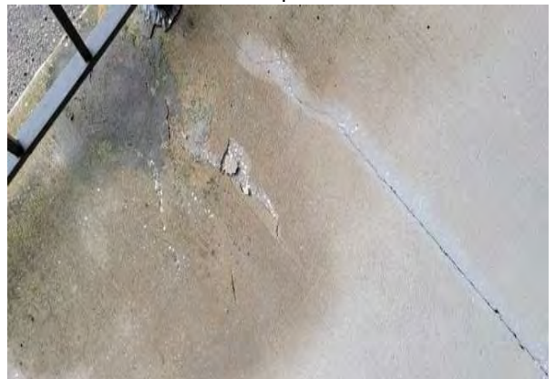
80 Spalled Concrete Near Unit 204
