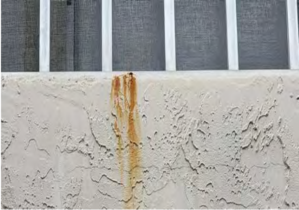
43 Unit 202 Rust at Balcony
