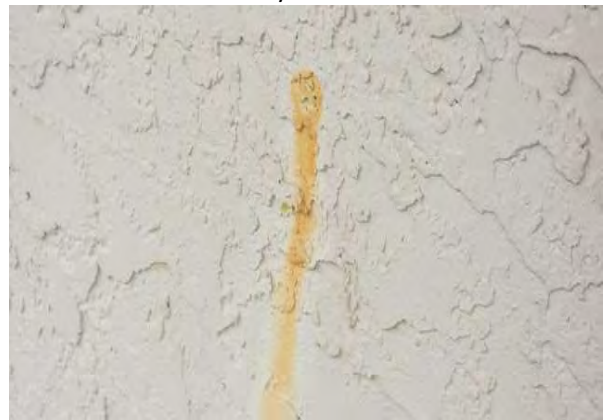
69 Rust at Wall Near Unit 206
