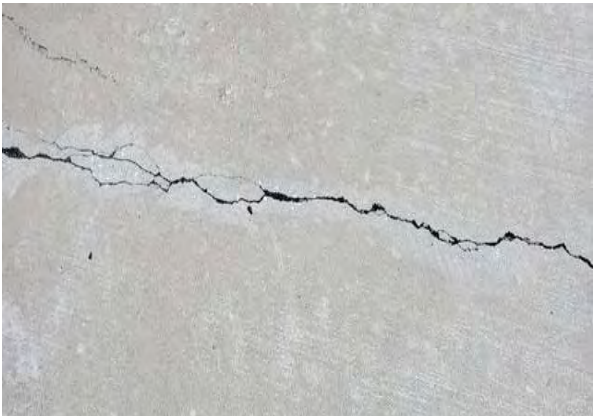
103 Cracked Walk Near Unit 305
