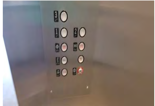
28 Elevator Control Panel
