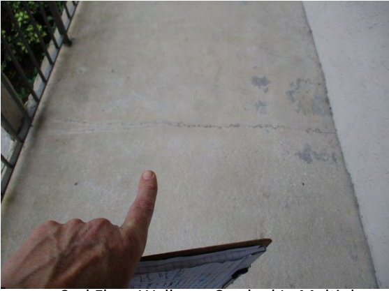
17 2nd Floor Walkway Cracked In Multiple Areas
