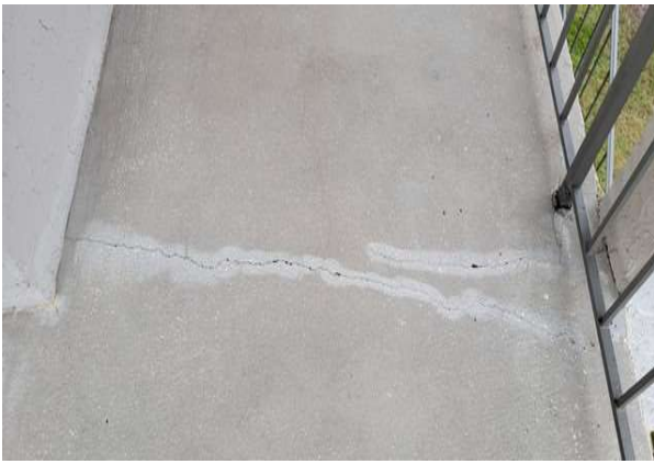
48 Crack in Walkway Near Unit 306
