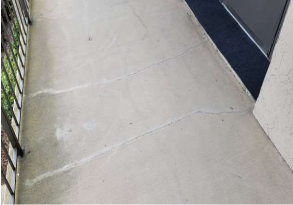
83 Cracked Walk Near Unit 203
