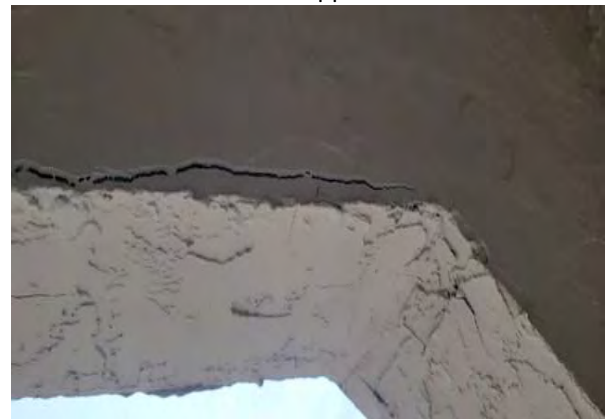
40 Unit 103 Cracked Support
