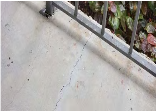
69 2nd Floor Right Staircase Cracked Walk
