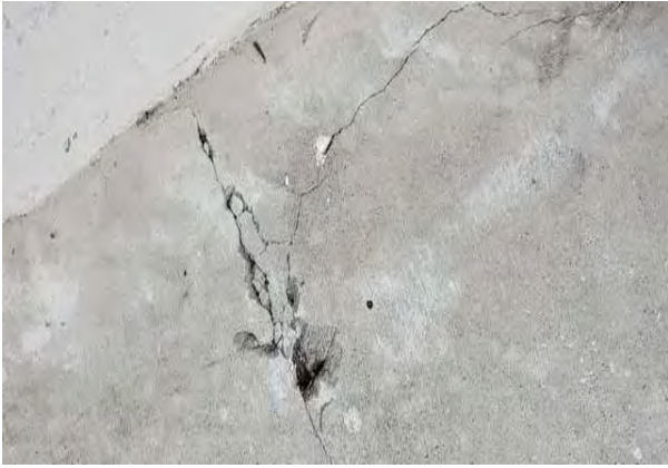
105 Spalled Concrete Near Unit 305
