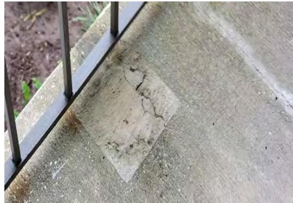
86 Failing repair Near Unit 202
