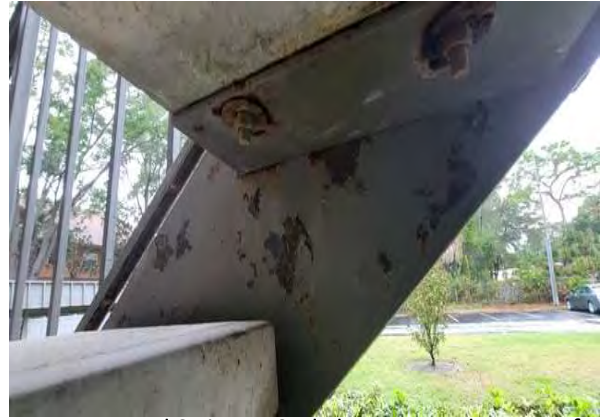
89 Rusted Stringer 2nd Floor to 1st Floor at Left Stairs
