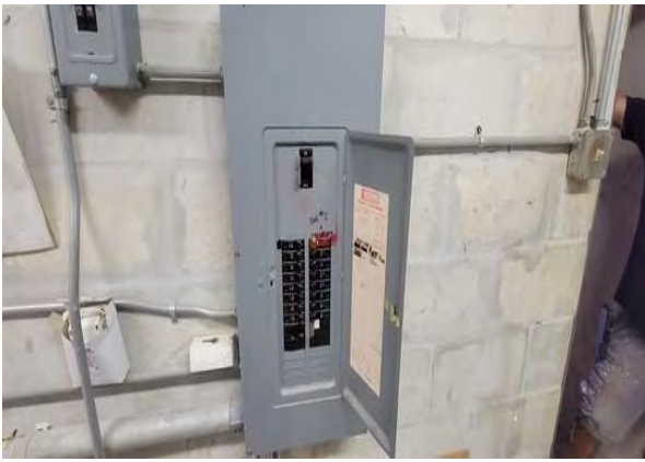
17 Electrical Panel Fire Alarm Room
