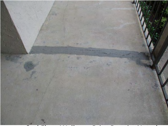
25 2nd Floor Walkway Prior Repairs Noted Throughout
