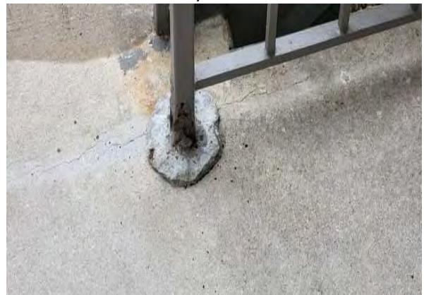
79 2nd Floor Rusted Handrail Left Stairs
