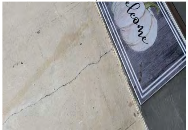
78 Cracked Walk Multiple Areas 2nd Floor
