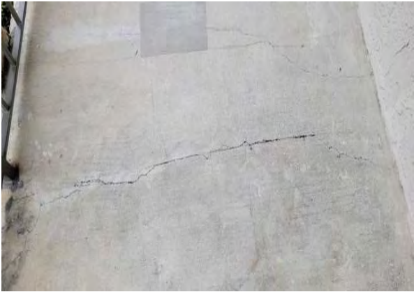
66 Crack in Walkway Near Unit 205
