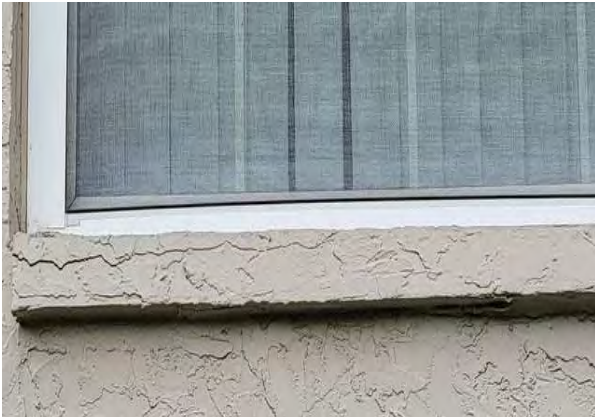
35 Unit 204 Cracked Sill
