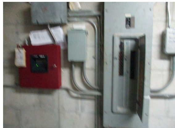
16 Sub Panels & Fire Control Panel
