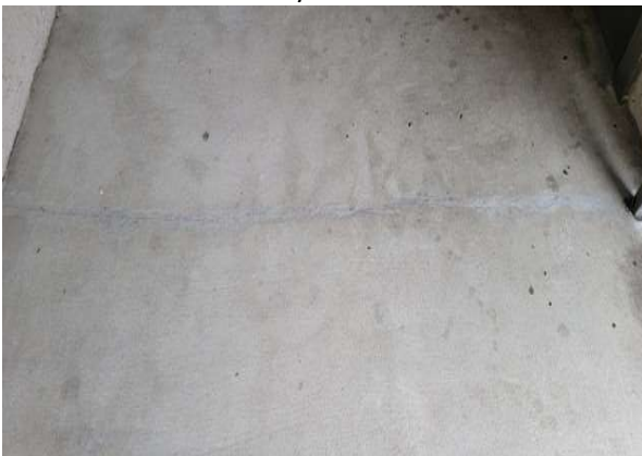
38 Cracked Walkway 3rd Floor Elevator Lobby
