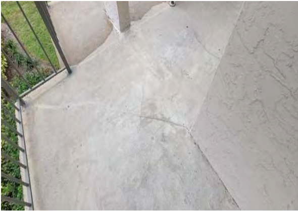
74 Crack in Walkway 2nd Floor Front Left Corner
