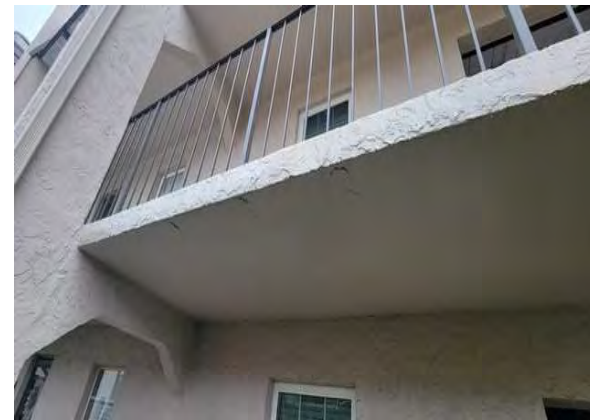
53 Cracked Walk Near Unit 106
