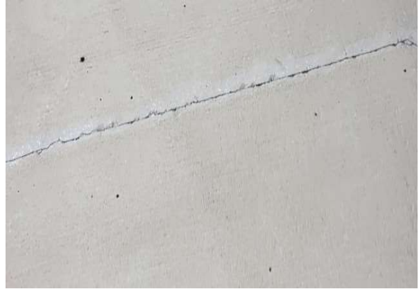
84 Cracked Walk Near Unit 203
