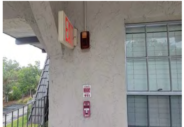
24 Fire Alarm Pullblock and Siren Overview
