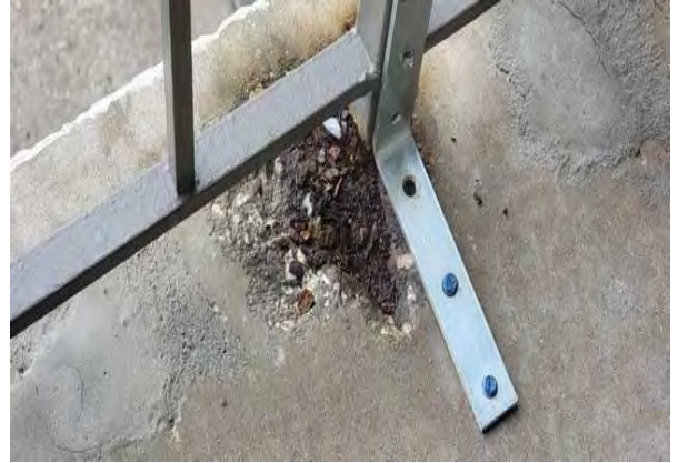
100 Spalled Concrete Ner Unit 304
