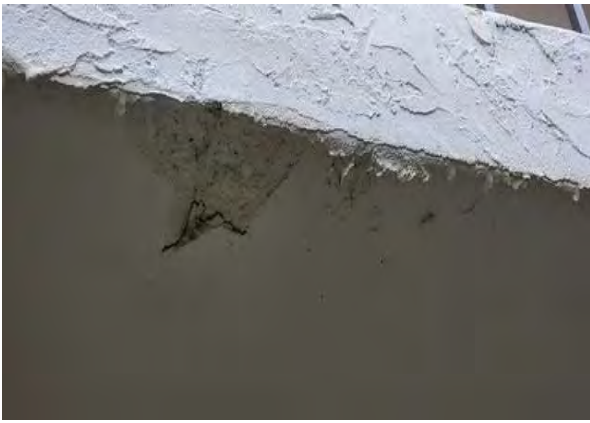
49 Cracked Walk Above Unit 102
