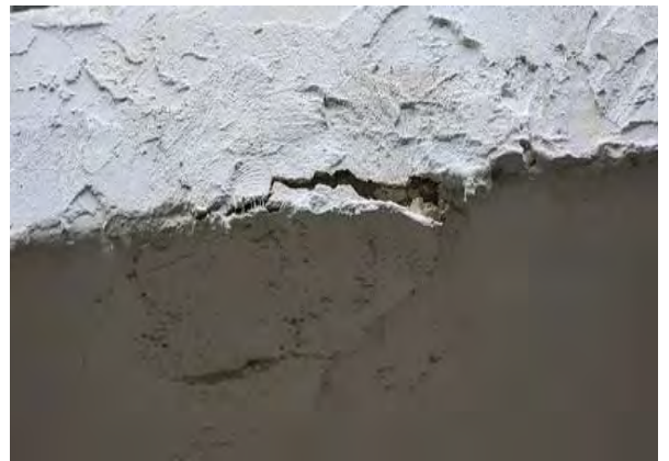
46 Cracked Walk Above Unit 102
