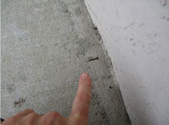
11 3rd Floor Walkway Concrete Spalling With Rebar Exposed & Corroded Multiple Areas
