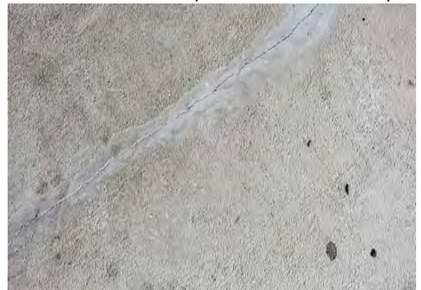
39 Cracked Walkway 3rd Floor Elevator Lobby
