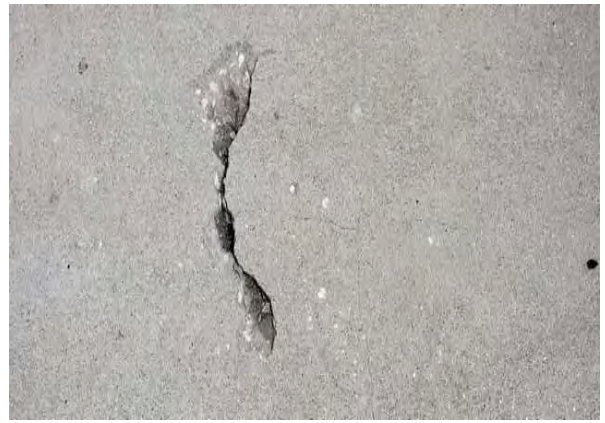
57 Spalled Concrete 2nd Floor Near Right Stairs
