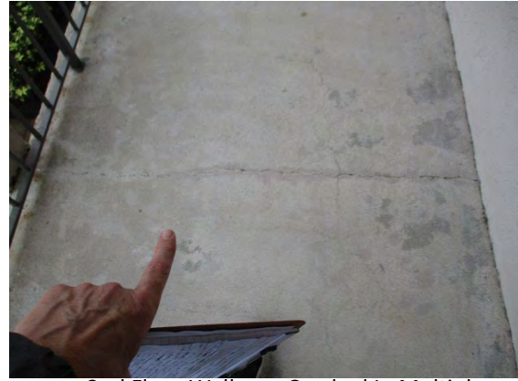
18 2nd Floor Walkway Cracked In Multiple Areas
