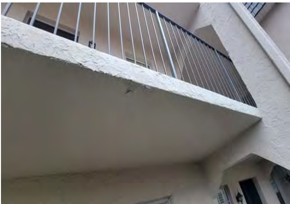
47 Cracked Walk Above Unit 102
