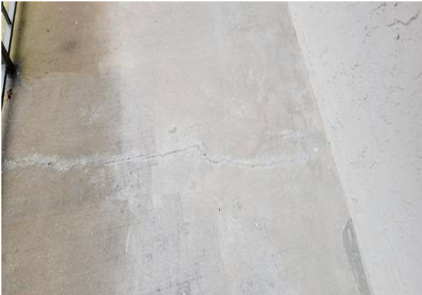
75 Cracked Walk Multiple Areas 2nd Floor
