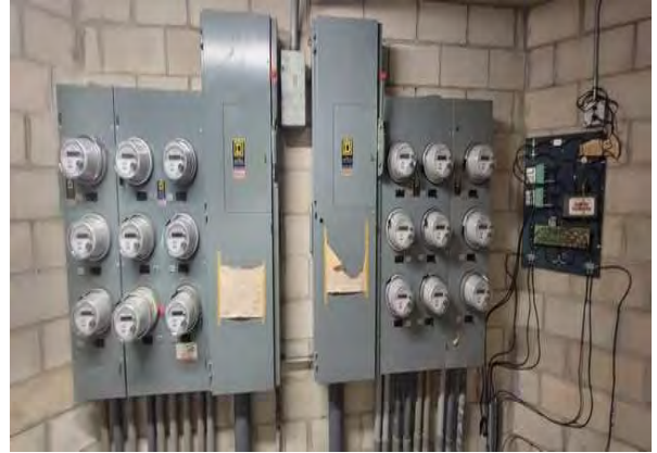
12 Meter Banks and Disconnects
