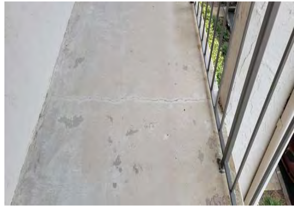
94 Cracked Walk Near Unit 301
