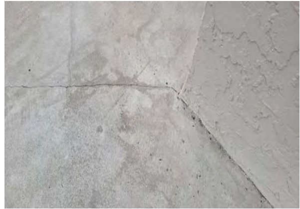
75 Crack in Walkway 2nd Floor Front Left Corner
