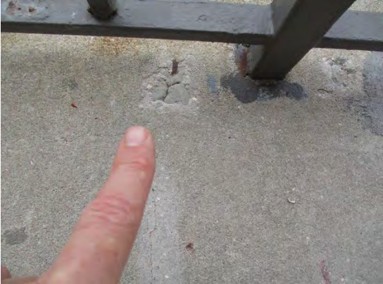
19 2nd Floor Walkway Concrete Spalling with Exposed Rebar (Corroded) Multiple Areas
