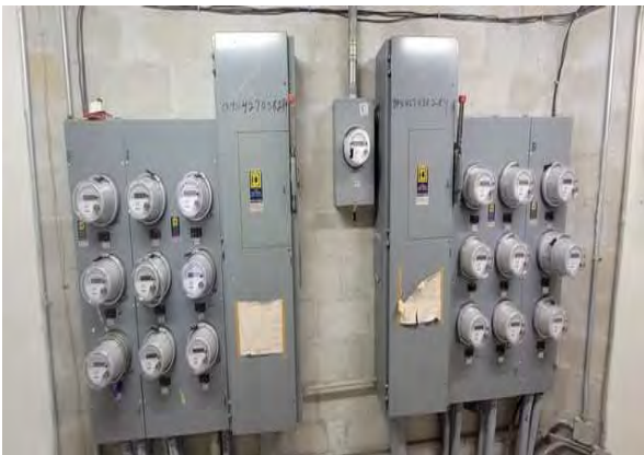
15 Meter Banks and Disconnects
