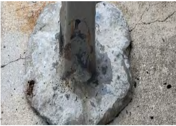
80 2nd Floor Rusted Handrail Left Stairs
