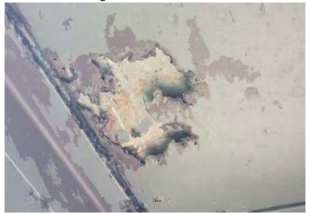
62 Rusted Right Staircase 1st Floor
