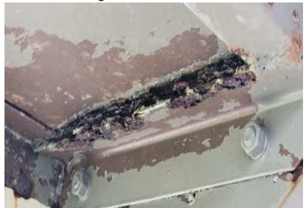
64 Rusted Right Staircase 1st Floor
