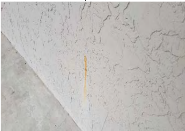
68 Rust at Wall Near Unit 206
