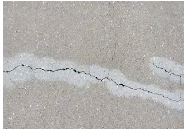
49 Crack in Walkway Near Unit 306
