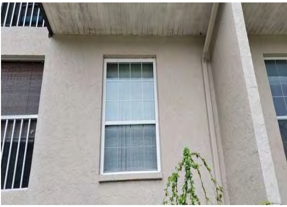
33 Unit 204 Cracked Sill
