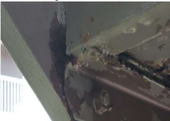
63 Rusted Right Staircase 1st Floor
