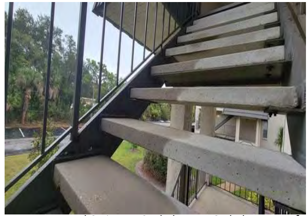
81 Rusted Stringer 2nd Floor to 3rd Floor at Left Stairs
