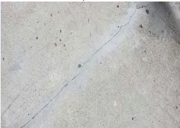
44 Crack in Walkway Near Unit 304
