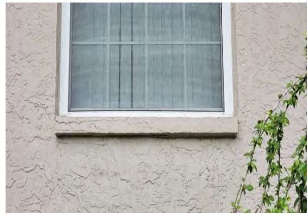
34 Unit 204 Cracked Sill
