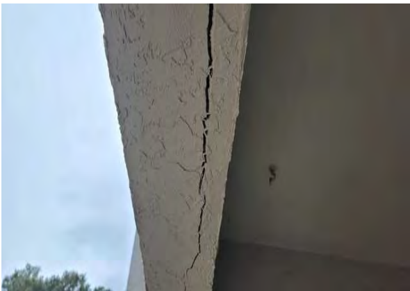
37 Unit 103 Cracked Support
