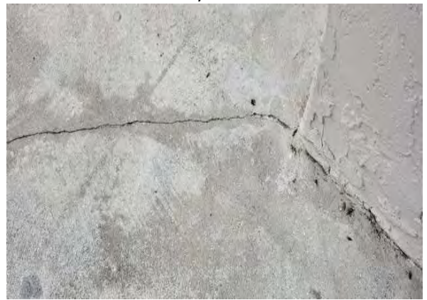
77 Crack in Walkway 2nd Floor Front Left Corner
