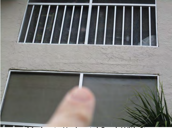
35 Moderate Horizontal Crack With Stucco Bulging Rear Left Side of Building
