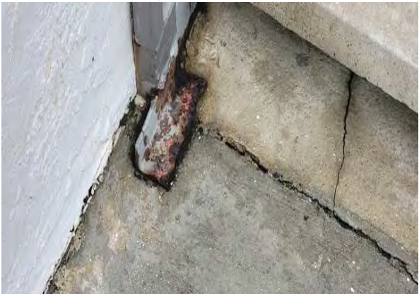
71 2nd Floor Right Staircase Rusted Bracket
