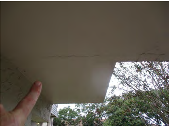
29 1st Floor Walkway Ceiling Prior Repair With Displacement Left Side of Building
