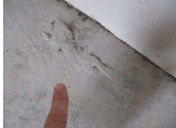
12 3rd Floor Walkway Concrete Spalling Multiple Areas
