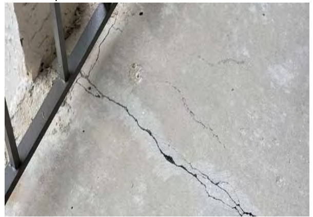
102 Cracked Walk Near Unit 305
