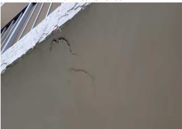
55 Cracked Walk Near Unit 106
