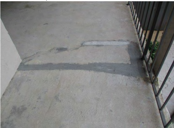
23 2nd Floor Walkway Prior Repairs Noted Throughout
