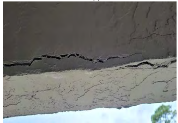
38 Unit 103 Cracked Support
