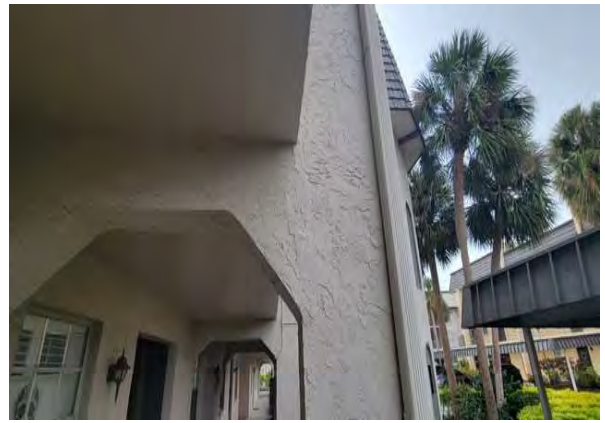
50 Crack in Wall Near Unit 103
