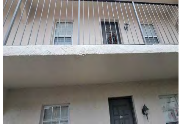
44 Cracked Walk Above Unit 102
