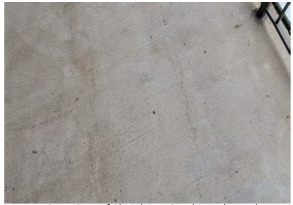
41 Overview of Shrinkage Cracking Throughout Building
