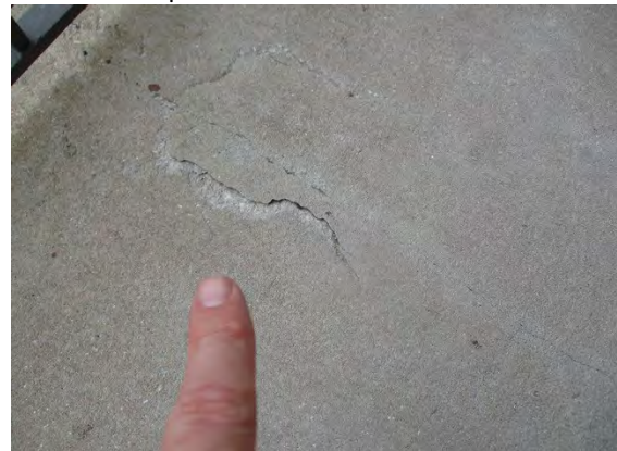
22 2nd Floor Walkway Concrete Spalling Multiple Areas
