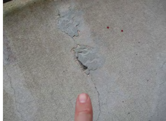
20 2nd Floor Walkway Concrete Spalling Multiple Areas
