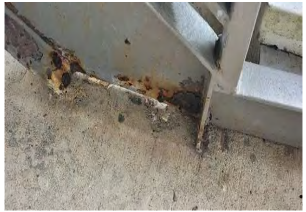
58 Rusted Stringer Right Staircase 1st Floor
