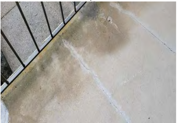
79 Spalled Concrete Near Unit 204
