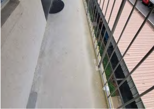
91 Spalled Concrete Near Unit 301
