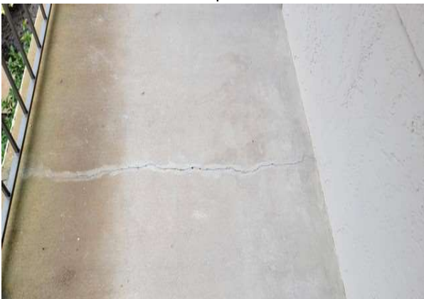
77 Cracked Walk Multiple Areas 2nd Floor
