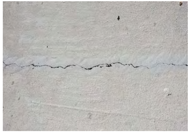
98 Cracked Walk Near 3rd Floor Elevator
