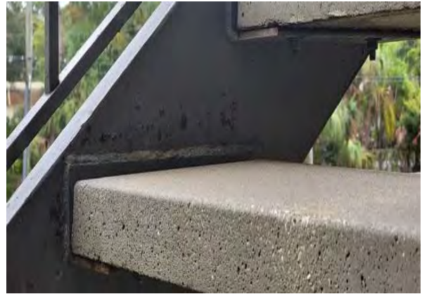
83 Rusted Stringer 2nd Floor to 3rd Floor at Left Stairs
