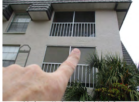
34 Moderate Horizontal Crack With Stucco Bulging Rear Left Side of Building
