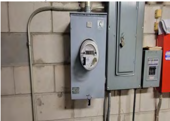
13 Electrical Room Meter
