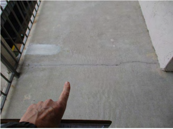
9 3rd Floor Walkway Cracked In Multiple Areas
