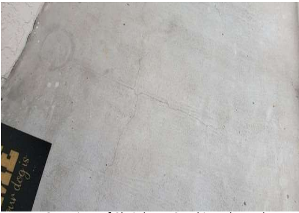
40 Overview of Shrinkage Cracking Throughout Building
