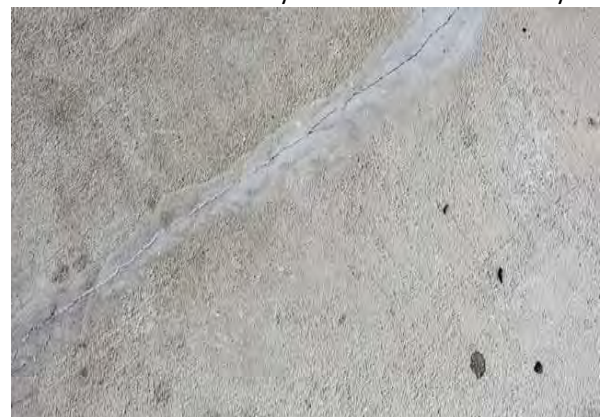
39 Cracked Walkway 3rd Floor Elevator Lobby
