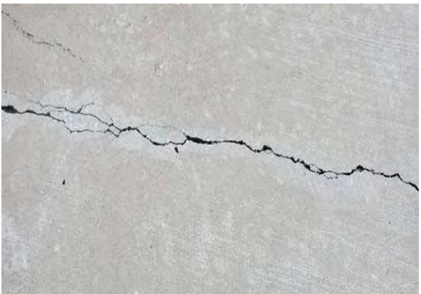
103 Cracked Walk Near Unit 305
