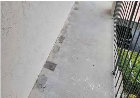
87 Failing Repairs to Walk 3rd Floor Near Left Stairs
