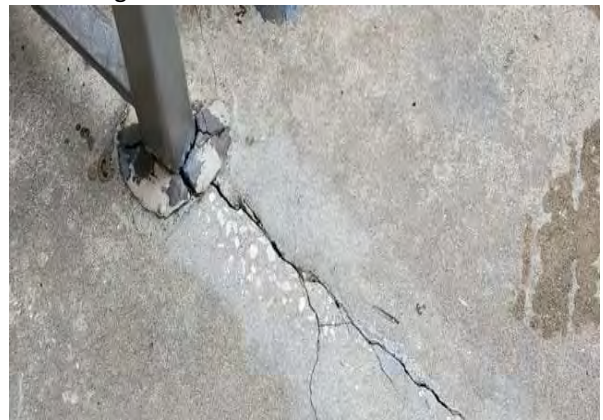
53 Crack in Walkway Base of Stairs 2nd Floor Right Side
