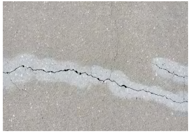
49 Crack in Walkway Near Unit 306
