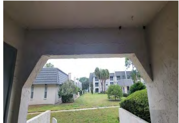
36 Unit 103 Cracked Support
