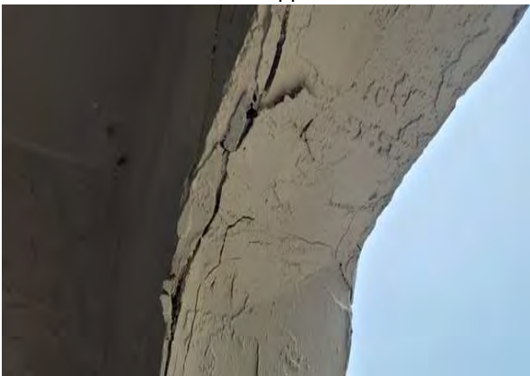
39 Unit 103 Cracked Support
