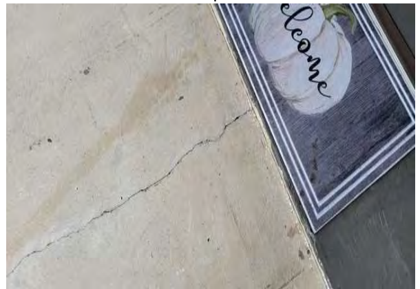
78 Cracked Walk Multiple Areas 2nd Floor
