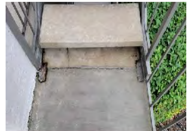
70 2nd Floor Right Staircase Rusted Bracket
