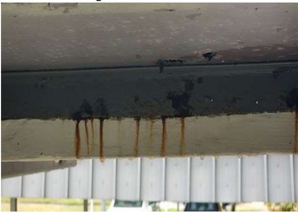
61 Rusted Right Staircase 1st Floor
