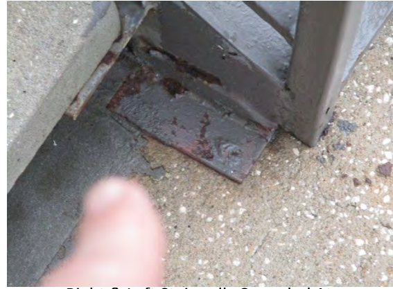
26 Right & Left Stairwells Corroded At Connection Points
