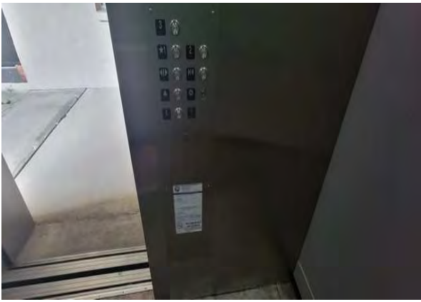
25 Elevator Control Panel
