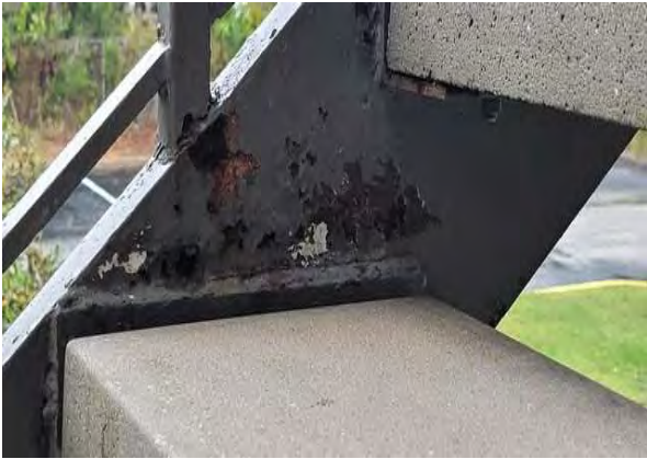
82 Rusted Stringer 2nd Floor to 3rd Floor at Left Stairs
