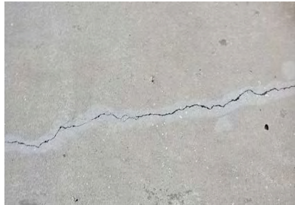
96 Cracked Walk Near Unit 301
