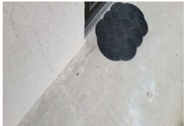
104 Spalled Concrete Near Unit 305
