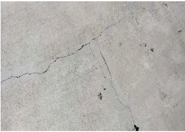
72 Crack in Walkway Near Unit 204
