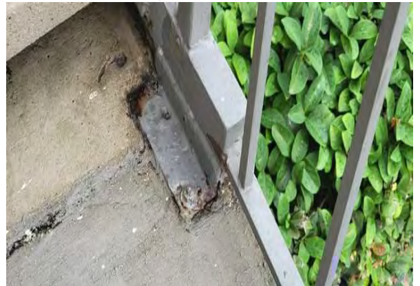
72 2nd Floor Right Staircase Rusted Bracket
