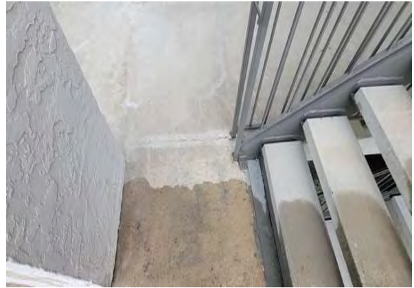
51 Crack in Walkway Base of Stairs 2nd Floor Right Side
