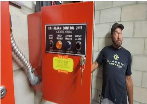
15 Fire Alarm Control Unit
