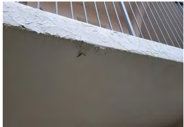
48 Cracked Walk Above Unit 102
