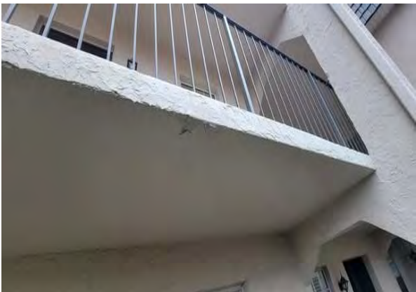
47 Cracked Walk Above Unit 102
