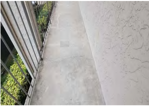
64 Crack in Walkway Near Unit 205
