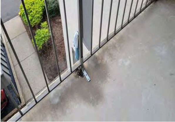
99 Spalled Concrete Ner Unit 304
