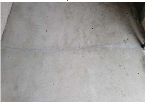
38 Cracked Walkway 3rd Floor Elevator Lobby
