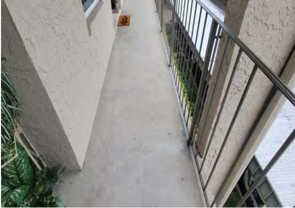
42 Crack in Walkway Near Unit 304
