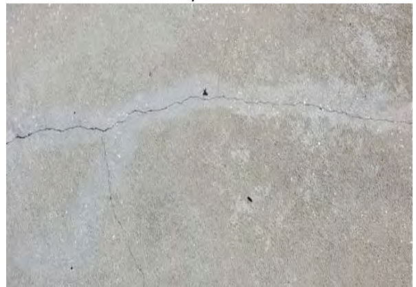
63 Crack in Walkway Near Unit 206
