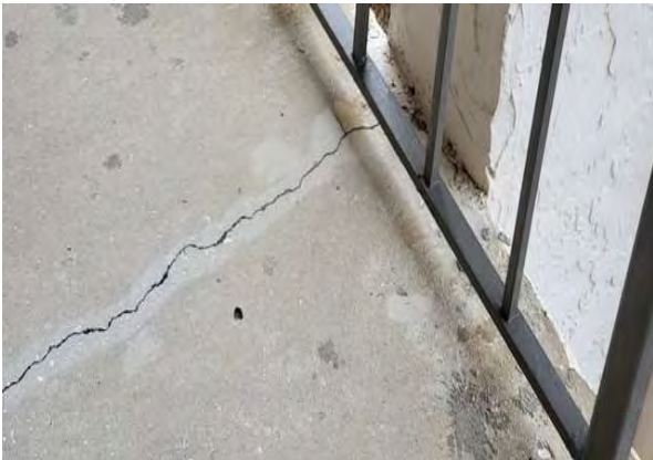
95 Cracked Walk Near Unit 301
