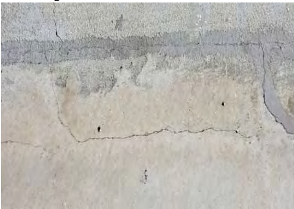
60 Crack in Walkway 2nd Floor Stairs Down Right Side
