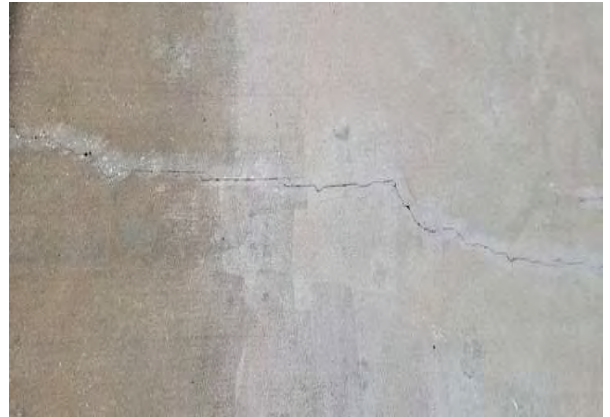
76 Cracked Walk Multiple Areas 2nd Floor
