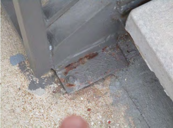
27 Right & Left Stairwells Corroded At Connection Points
