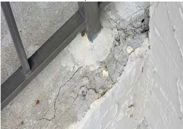
36 Cracked Walkway Near 303
