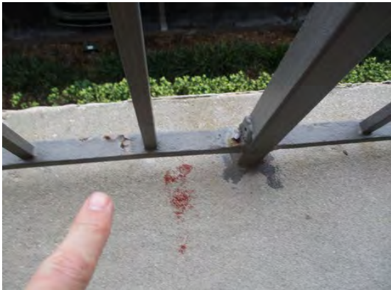
5 3rd Floor Railing Corroded In Multiple Areas
