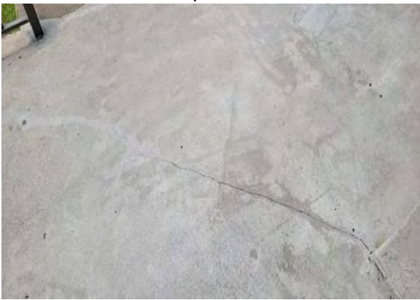
76 Crack in Walkway 2nd Floor Front Left Corner
