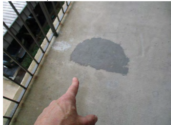
14 3rd Floor Walkway Prior Repairs Noted Throughout
