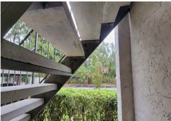
86 Rusted Stringer 2nd Floor to 1st Floor at Left Stairs
