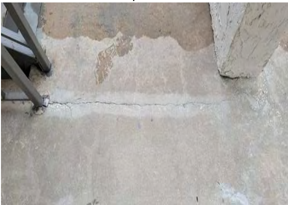
52 Crack in Walkway Base of Stairs 2nd Floor Right Side
