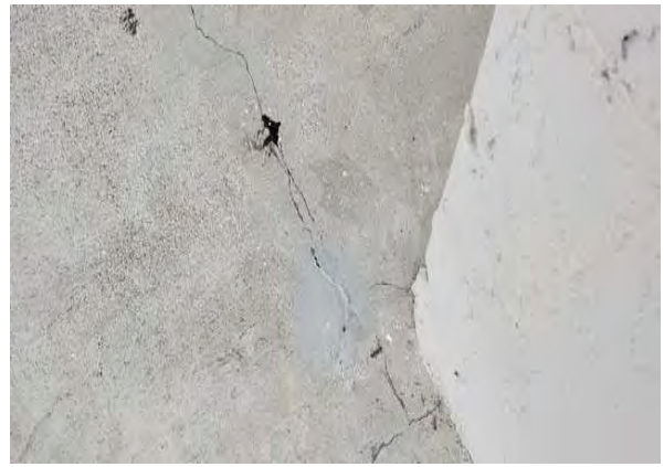
73 Crack in Walkway Near Unit 204
