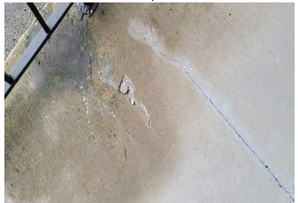
80 Spalled Concrete Near Unit 204
