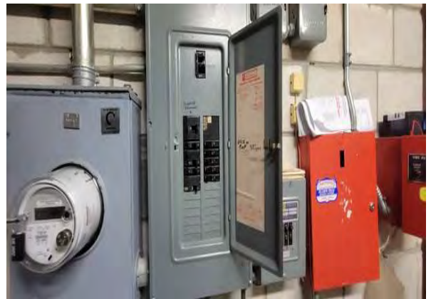
14 Electrical Room Panel
