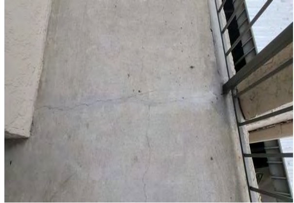
43 Crack in Walkway Near Unit 304
