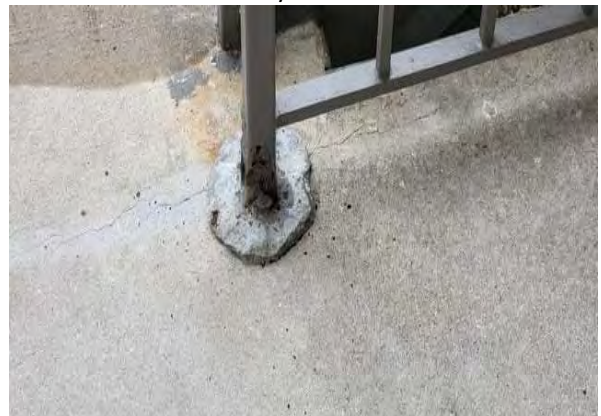
79 2nd Floor Rusted Handrail Left Stairs
