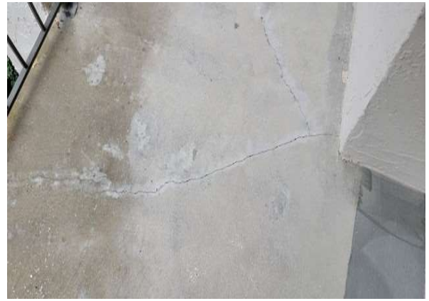
74 Cracked Walk Multiple Areas 2nd Floor
