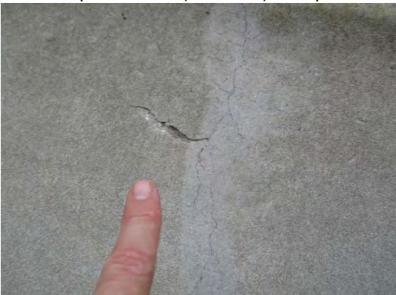
21 2nd Floor Walkway Concrete Spalling Multiple Areas
