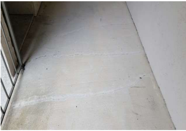
81 Cracked Walk Near 2nd Floor Elevator Door
