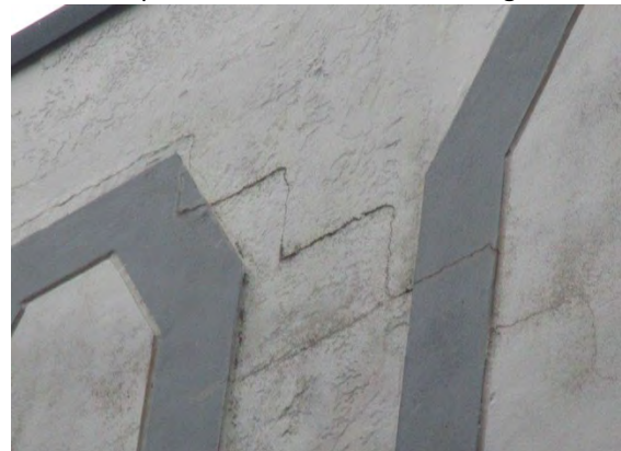
32 Moderate Step Crack With Displacement Rear of Building
