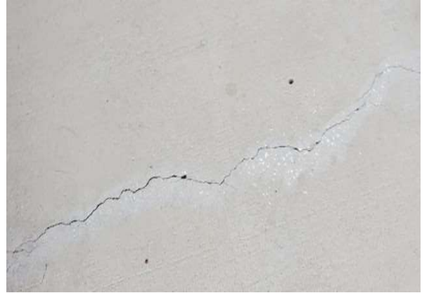
68 2nd Floor Right Staircase Cracked Walk
