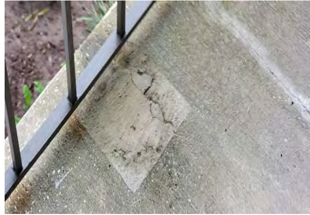
86 Failing repair Near Unit 202
