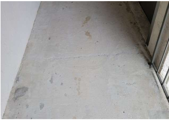
97 Cracked Walk Near 3rd Floor Elevator
