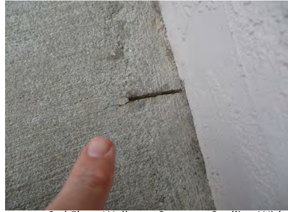
10 3rd Floor Walkway Concrete Spalling With Rebar Exposed & Corroded Multiple Areas
