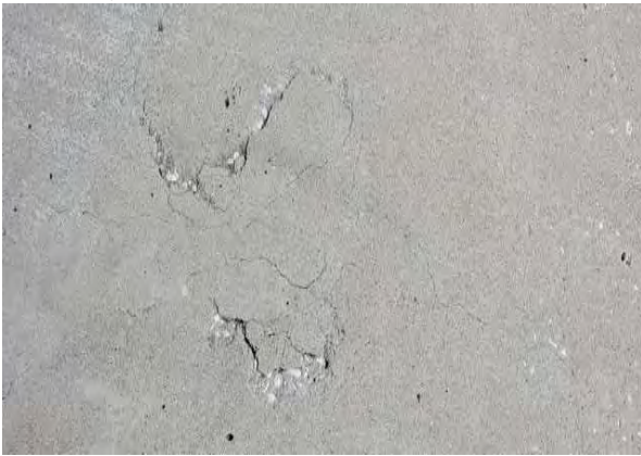
93 Spalled Concrete Near Unit 301
