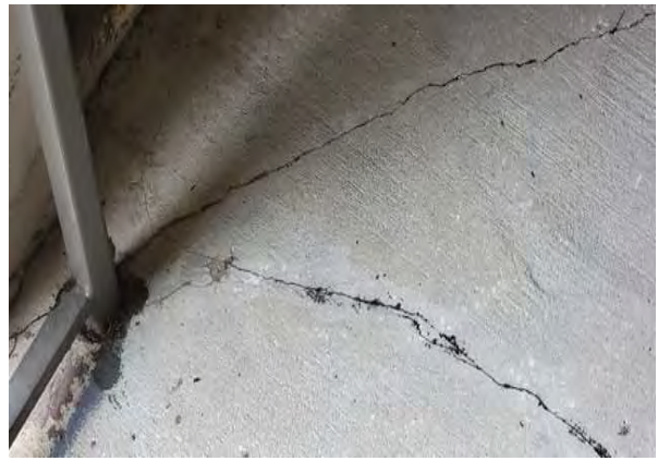
82 Cracked Walk Near 2nd Floor Elevator Door
