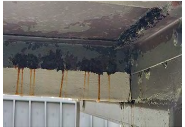
60 Rusted Right Staircase 1st Floor
