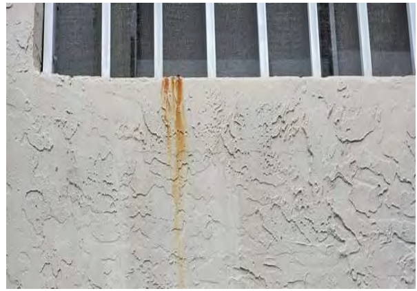
42 Unit 202 Rust at Balcony
