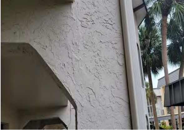
51 Crack in Wall Near Unit 103
