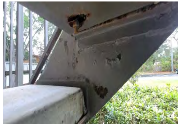
87 Rusted Stringer 2nd Floor to 1st Floor at Left Stairs
