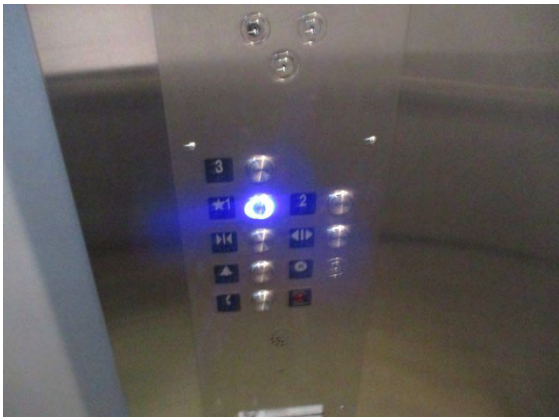
9 Elevator Cab Control Panel
