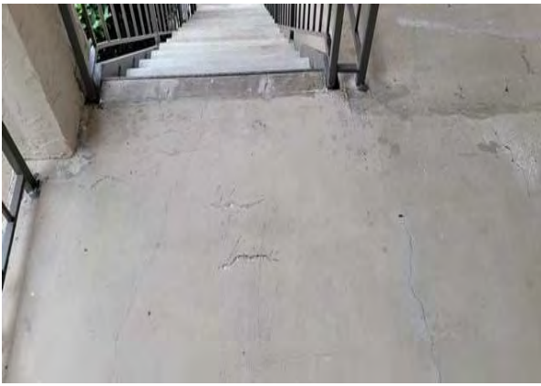
65 2nd Floor Right Staircase Spalled Concrete
