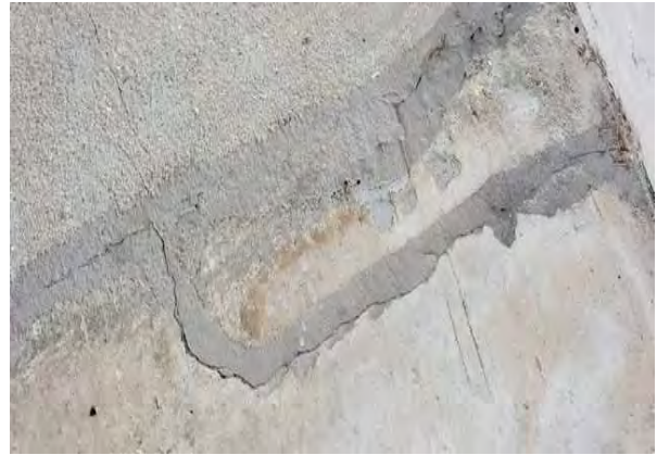
59 Crack in Walkway 2nd Floor Stairs Down Right Side
