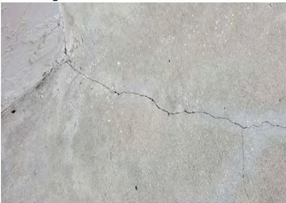
62 Crack in Walkway Near Unit 206
