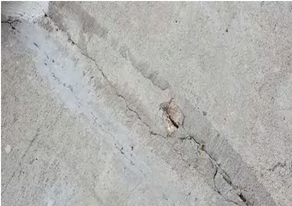
34 Cracked Walkway Near 303
