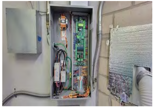
18 Elevator Control Board
