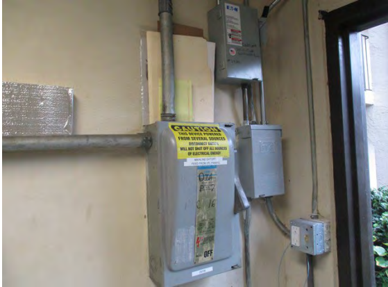
19 Main & Sub Panel
