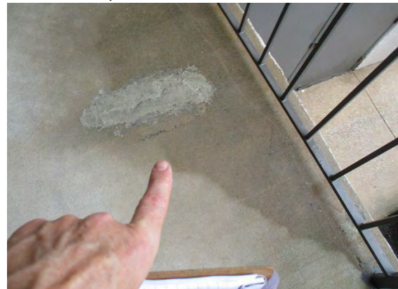
24 2nd Floor Walkway Prior Repairs Noted Throughout
