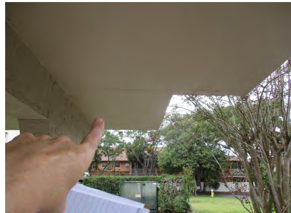
30 1st Floor Walkway Ceiling Prior Repair With Displacement Left Side of Building
