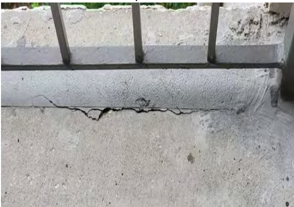
46 Crack in Walkway Near Unit 304
