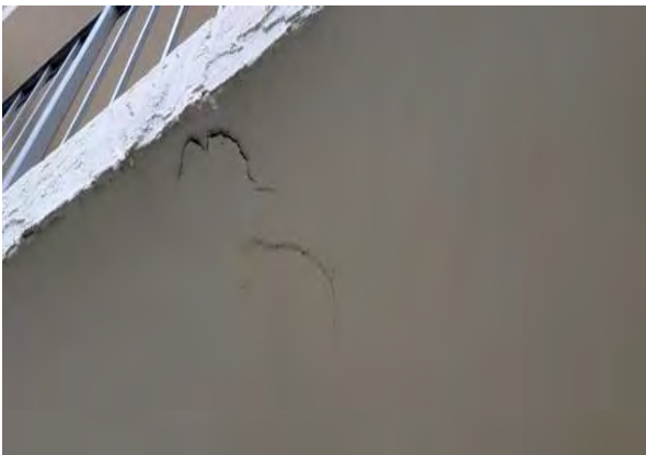
55 Cracked Walk Near Unit 106
